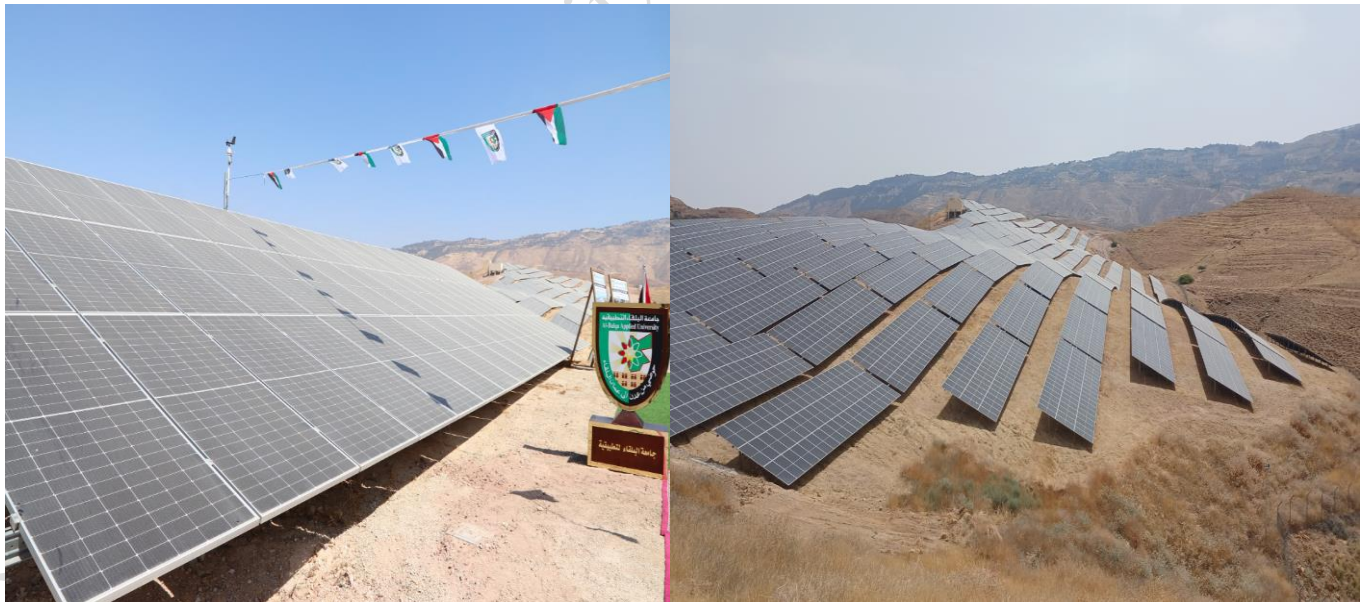
BAU's Solar park project with capacity 7MW
